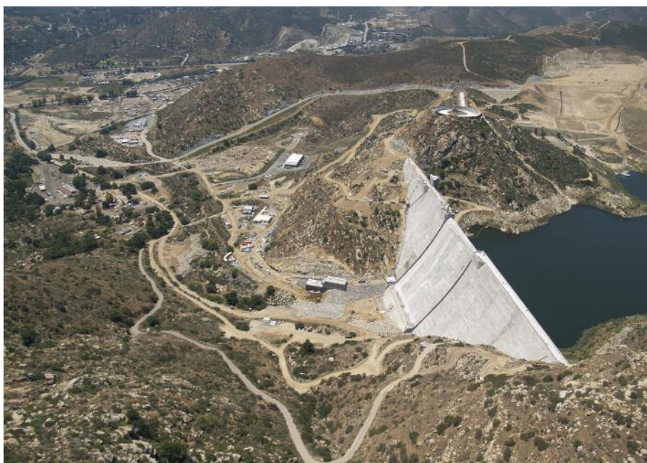
Pictured in the top right corner is the source of the aggregate for the RCC and the location of the future marina.
