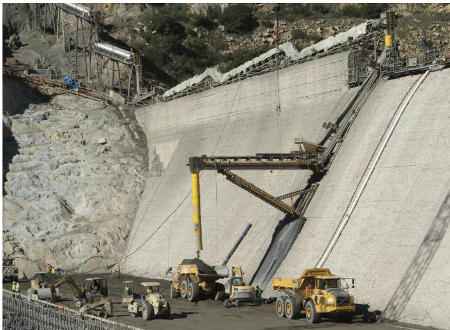
A conveyer system was used to transfer the RCC from the onsite batch plant to the dam.
