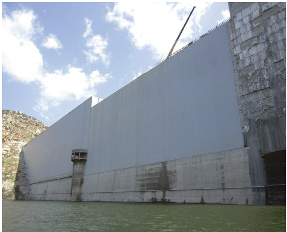
The San Vicente Dam was raised 117ft (35.7m), the highest dam raise in the U.S. and tallest dam raising use RCC in the world. Visible in the center of the dam is the original control tower. The raised dam section shows the upstream Carpi geomembrane liner.
