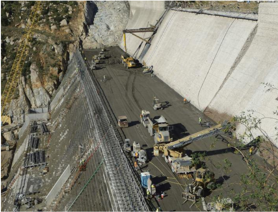
The RCC placement proceeded nearly continuously, enabling the contractor to work on the RCC immediately after it is laid, allowing the 600,000 cubic yards of dam raise concrete placement to be completed in less than a year.
